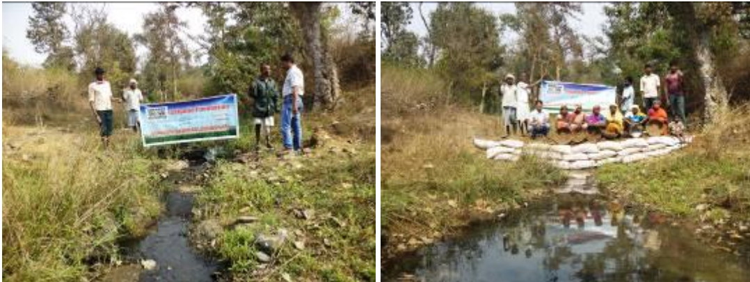
Check dam site at Dala nallah before our programme (left) and after (right)
