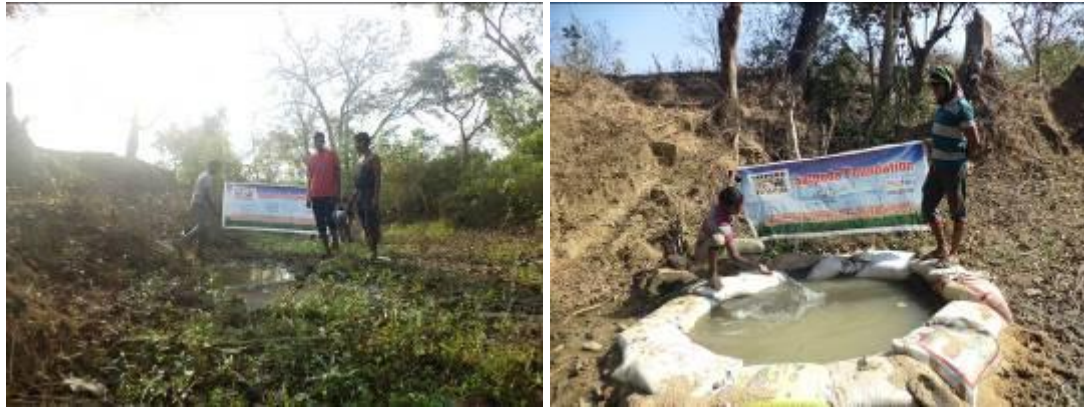
Water-tank site at Budbudi nallah before (left) and after our programme (right)
