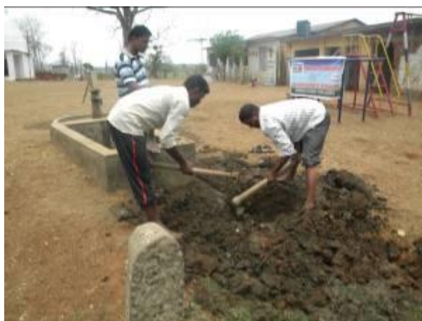
Volunteers clean area around hand pump and build soak pit at Jindatola
