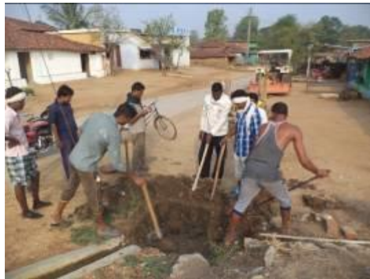
Villagers volunteer to dig a soak pit after cleaning area next to hand pump at Ghoti
