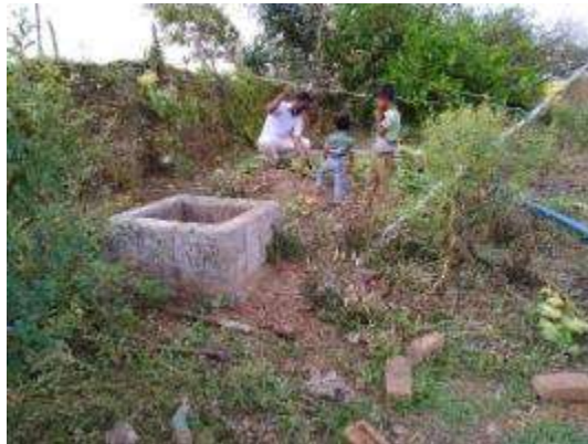
Aamajhiri – Niranjan undertaking repair of a faulty biogas unit
