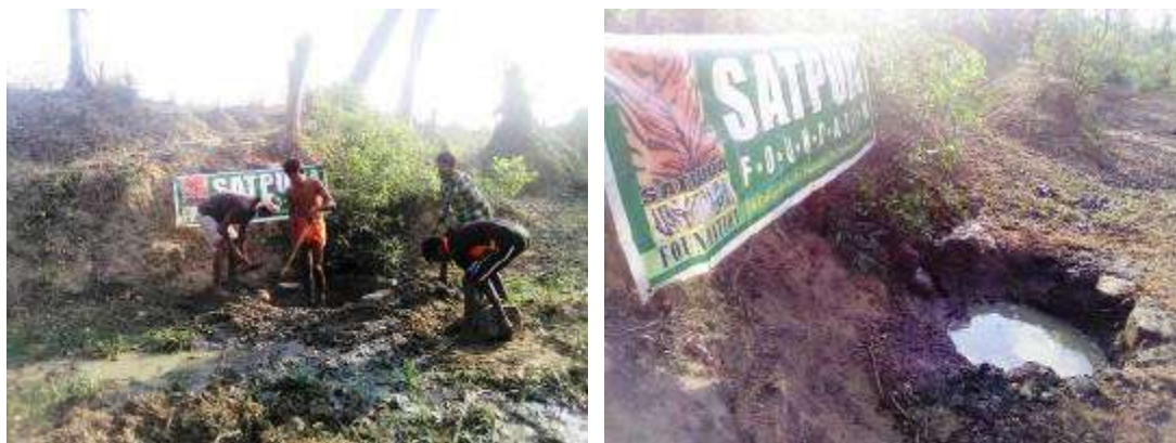
Chapri – Team prepares water hole at Budbudi Nallah (left); Waterhole completed (right)
